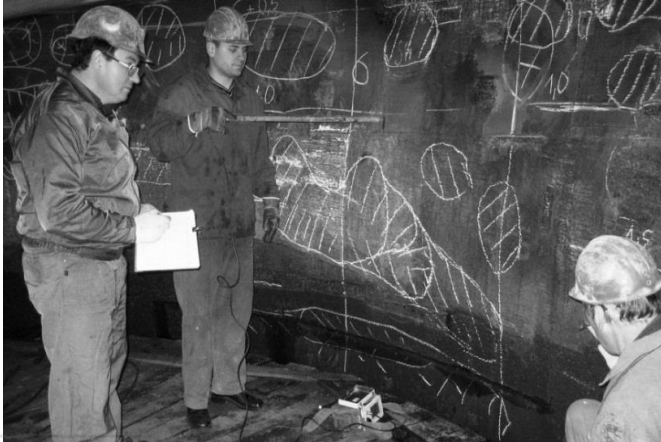
Fig. 16. The determination of the areas of poor contact of the metal to the reinforced concrete in the chamber of the working wheel of the hydraulic unit No. 12 of the hydroelectric power station in Kremenchug
