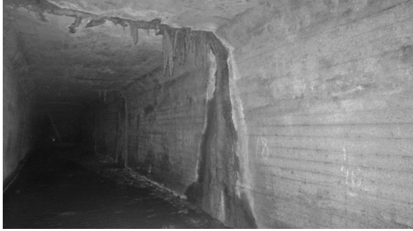
Fig. 13. The destroyed seams between individual slabs of support of sewer
