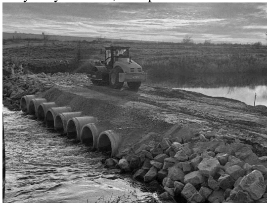
Fig. 1. Construction of a crossing over the Ingulets River connecting the village of Zarichne with Arkhangelsky of the Visokopil community [5]
