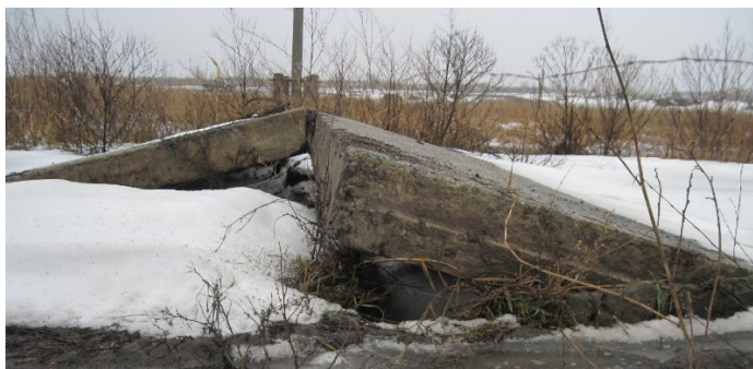
Fig. 1. The result of the impact of compression of the earth's surface on the concrete road pavement
