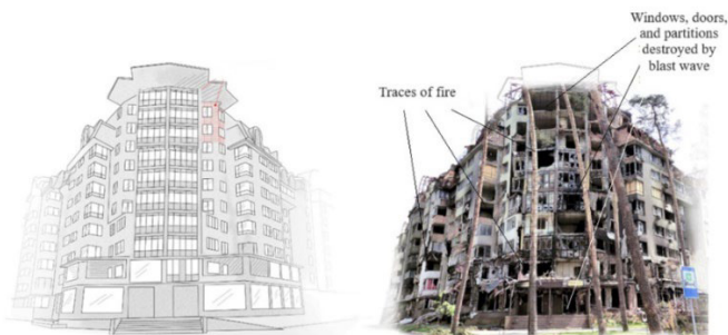
Fig. 10. Nature of damage and the scheme of destruction of the brick building of the "Ukraine" hotel in the city of Chernihiv
