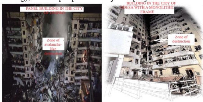
Fig. 12. Nature of damage to multi-story buildings: panel (left image) and reinforced concrete frame (right image)
