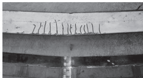
Fig. 3. The cracking pattern of composite steel beam strengthened with steel plate
